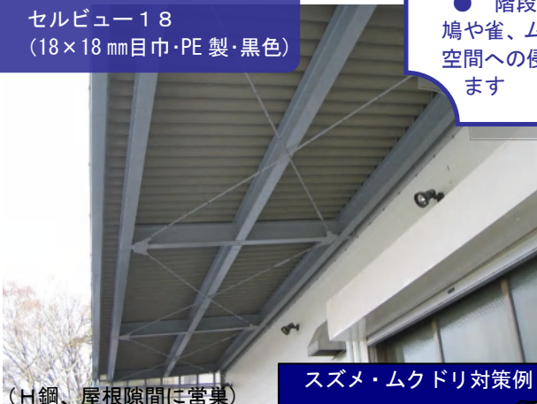
(H鋼、屋根隙間に営巣)
